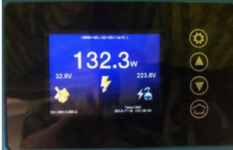
Main „Power View“ display during normal operation
