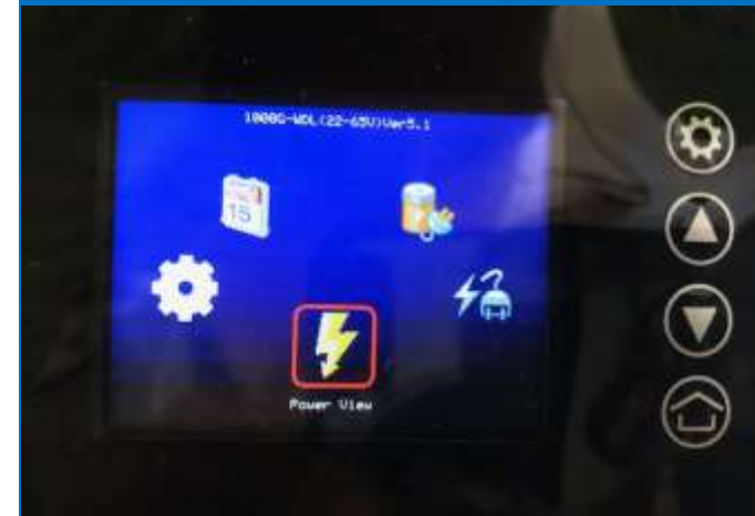
The inverter main menu
