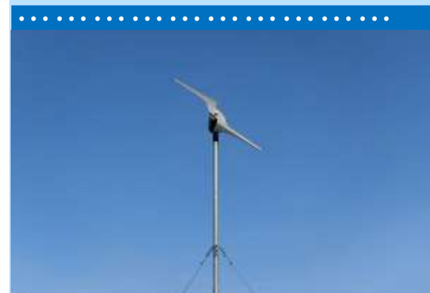
Stand-alone installation on a tower
