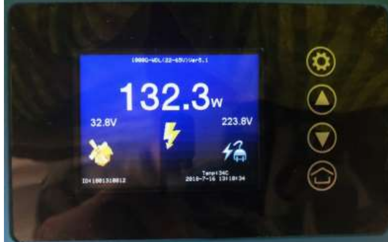
Main „Power View“ display during normal operation
